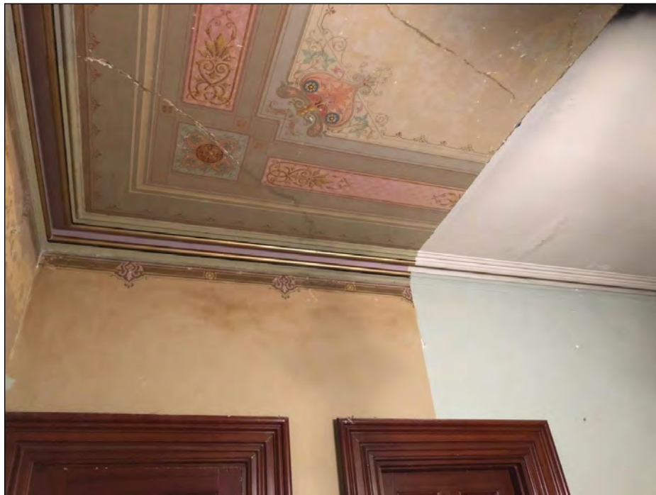
Restoration work at the John Hauck House in Cincinnati has uncovered original 1870s and 1880s intricate ceiling murals.
