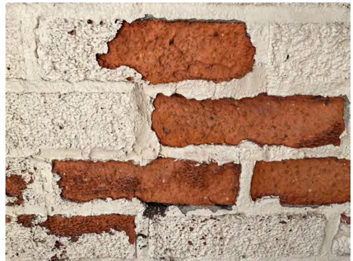
Masonry that has been painted resulting in trapped moisture and spalling of the brick.
